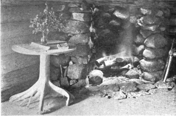
A Hearth with Many Cracks is Difficult to Keep Clean. The Standard of the Table is a Piece of Driftwood.
