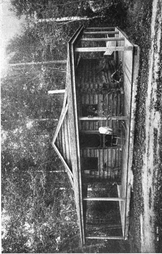
If the Roof is Very Flat in Regions of Heavy Snowfall, the Supporting Beams Should be Well Braced and of Stout Timbers.
